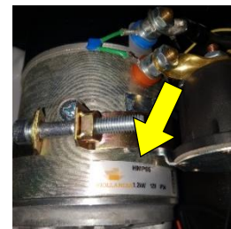
In the pump unit
